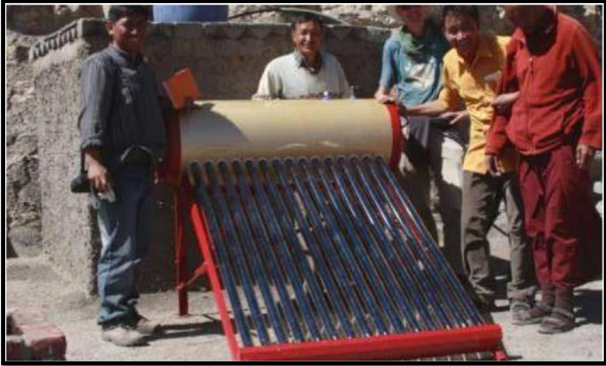
Installed Solar Heating System
